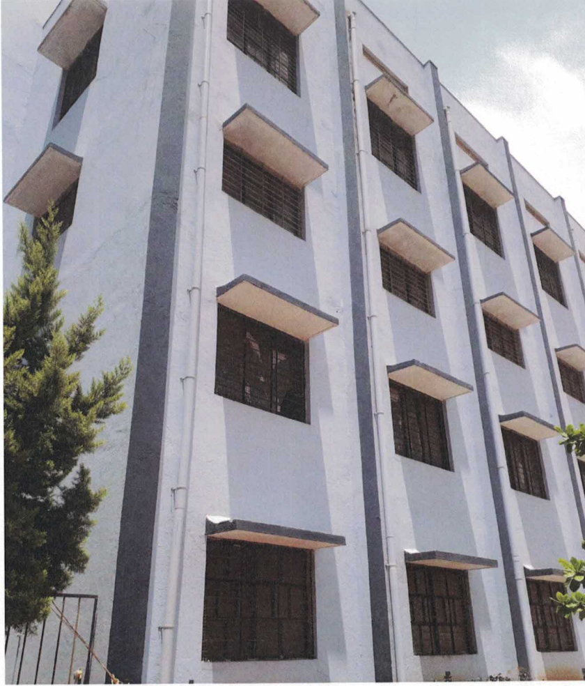
Down pipelines to collect and drain roof top water for ground recharging.
